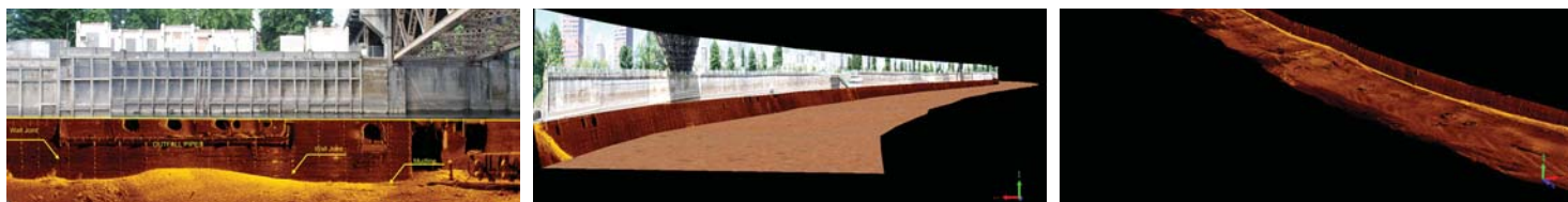
Sonar images combine with above-water photography to highlight infrastructure features of the harbor seawall along the Willamette River in Portland, Ore.
